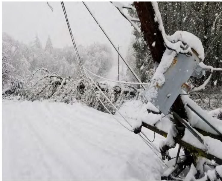
Figure 49 Downed Powerline due to Snowmageddon
